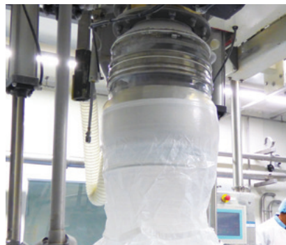
Bigbag station – inlet
